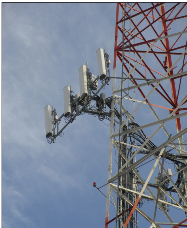
Figure 14. Cellular tower showing typical Remote Radio Head installation behind antennas at the tower top
